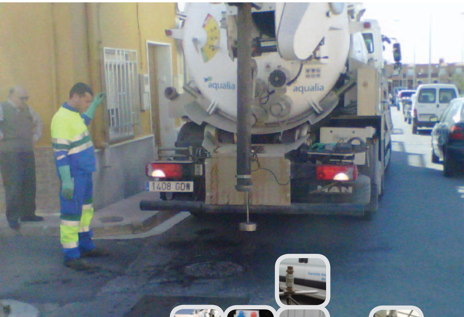
The sanitation trucks have an implementation installed that makes it possible to open heavy potholes.
